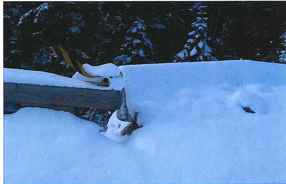
CK2361 Damaged delineator and guard rail
